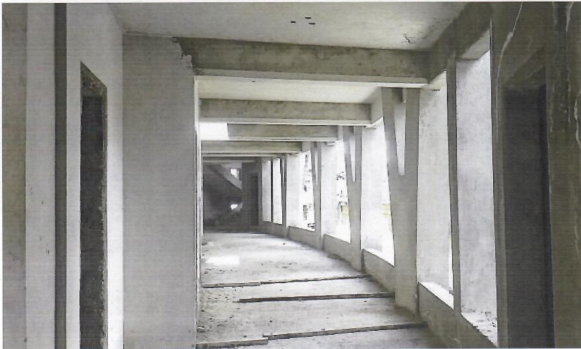
Image 6. View from the external corridors within the chamber. Plastering of walls ongoing.
