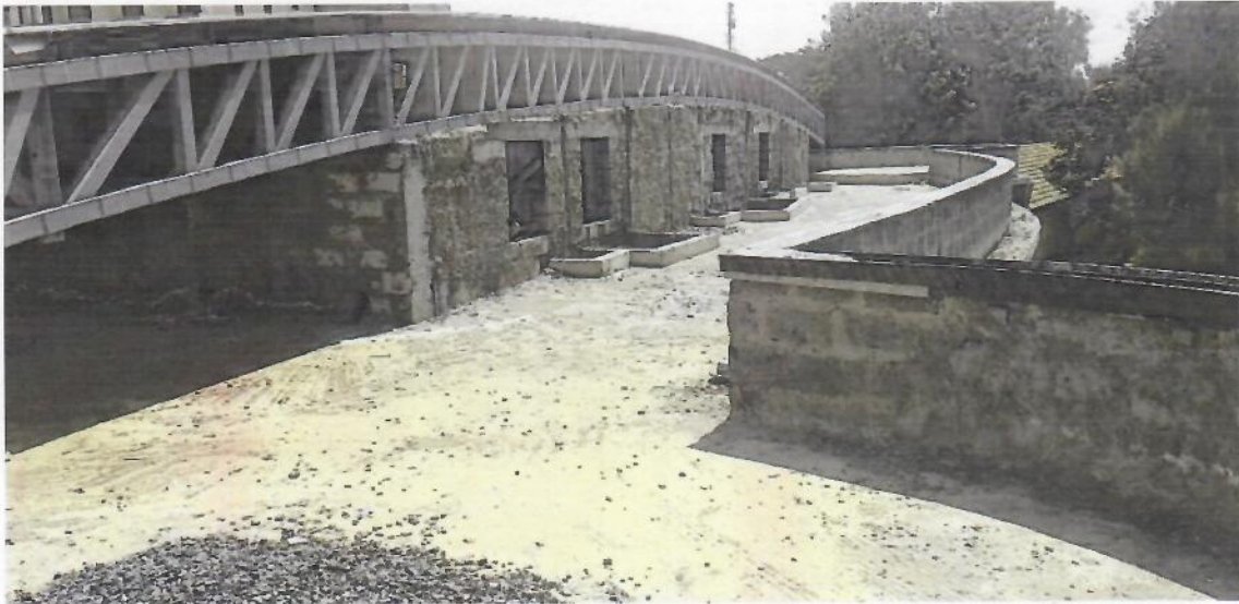
Image 5. View of the roof slab area, parapet wall done and steel fabrication and fixing done.
