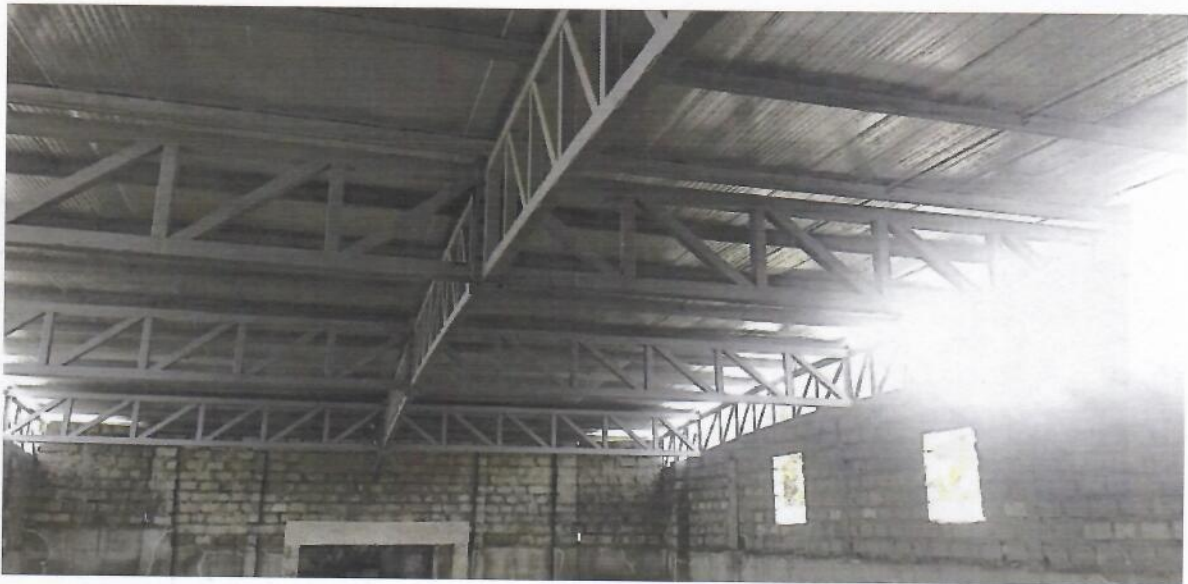
Image 4. View of some of the roof trusses fabricated on site at the roof level. Heat insulation and roof cover installed. Finishes to follow.
